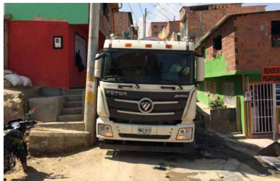
It is a complicated matter to do upgradings in the dense structure of Potosí. In this image, a street is being paved
