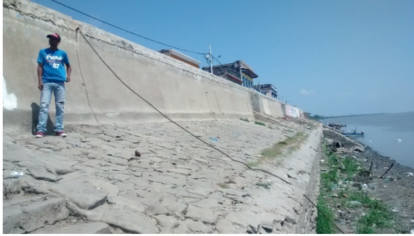
The Calamar wall that almost collapsed during the Ola Invernal
