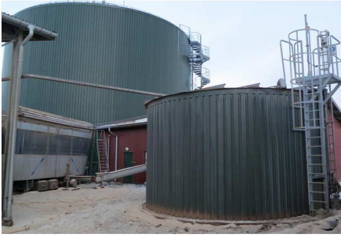
Figure 5: Lövsta biogas plant featuring pre-mixing tank (right) and digestion chamber
