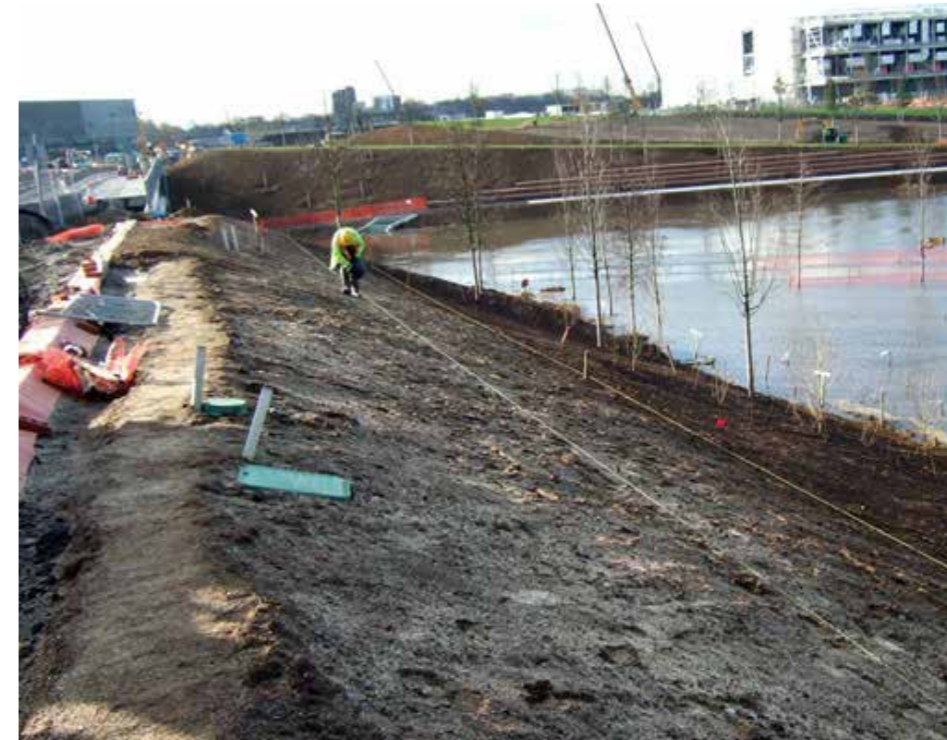
The Native Wildflower Garden under construction in January 2011. The top soil is removed and the plants are seeded. Photo: James Hitchmough, 2011
