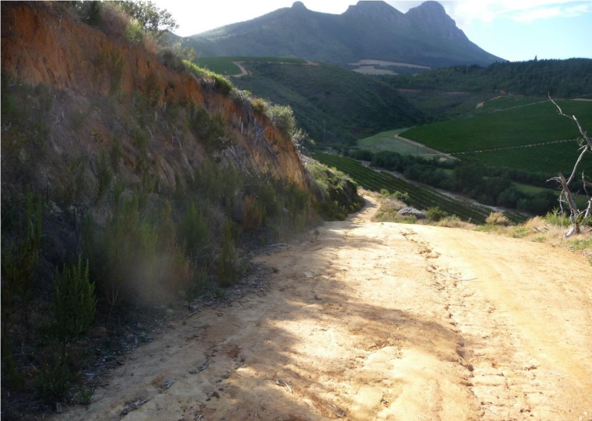
Figure 39 Excess water originating from block 510 and 511 is transported down the steep hillsides, seen to the left on this photo. Together with enormous water flows illustrated in figure 19 this water flow contributes to eroding of the road.
