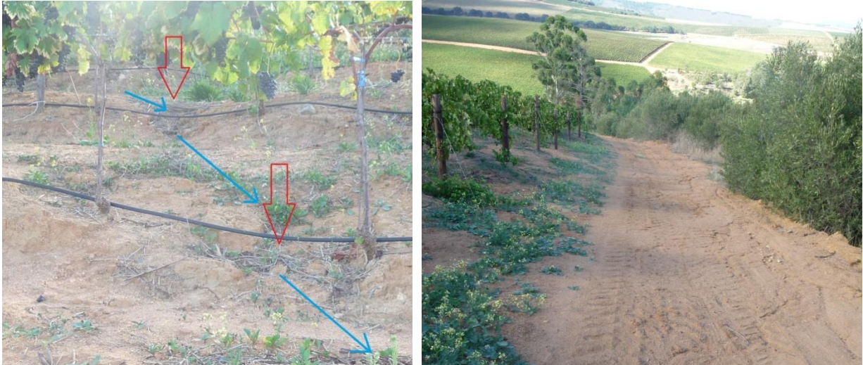
Figure 37 Signs of excess water flow on the south eastern side of block 510. Red arrows showing breakage of the forming terrace wall.
