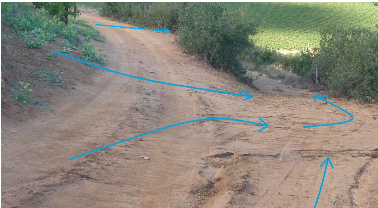
Figure 38 Three flows of excess water reunite to one major flow down the road leading to block 27 and 28.
