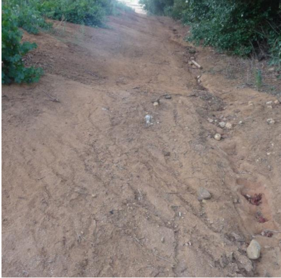
Figure 35 Runoff escaping the above channel and runoff from block 308 causing erosion on the road.
