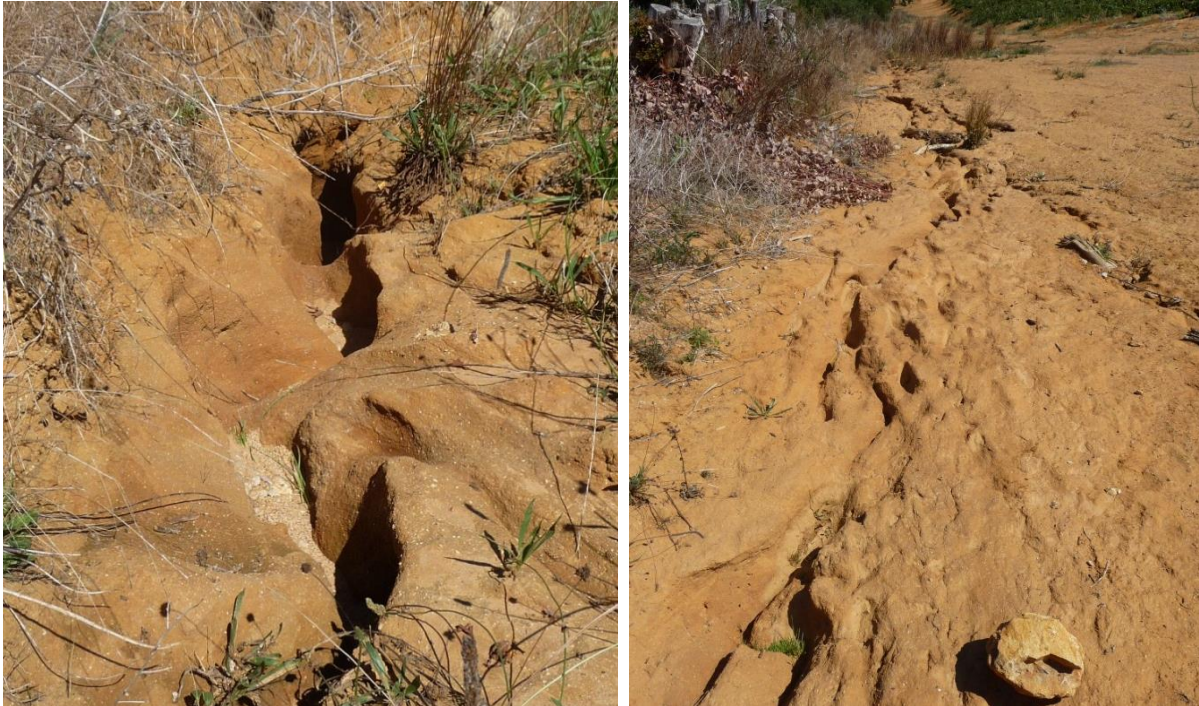
Figure33 Upper left: Waterway between block 310 and 410. Ending at the next crossroad. Upper right: Downslope the end of the waterway. Outlet pipe releasing water with great forces from large water flow create severe rill erosion. Lower left: Deep rills continuing downslope. Lower right: Rills eventually ending in the natural area, seen on the left side of the photo.
