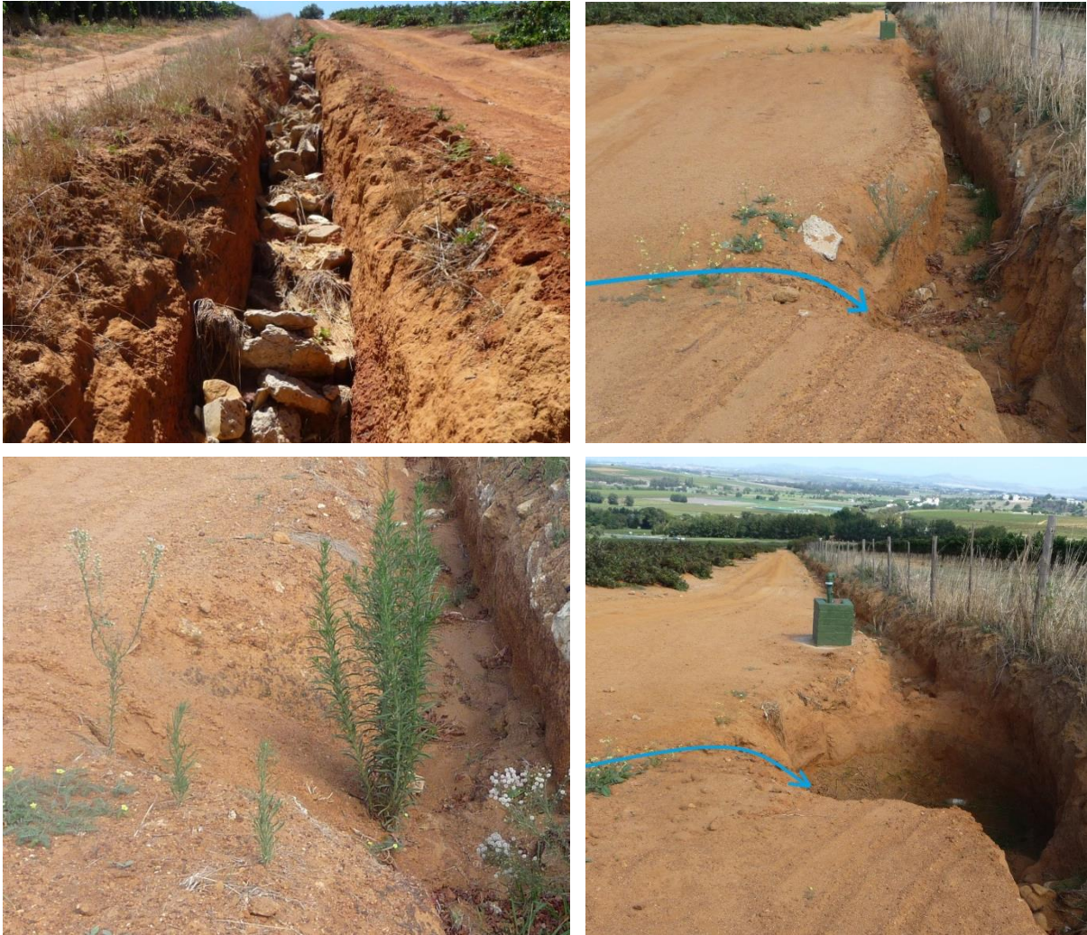
Figure 26 Open ditch at the western/northern vineyard border. Steep, vertical walls with poor vegetation cover, especially on the right side. The wall has collapsed in places.
