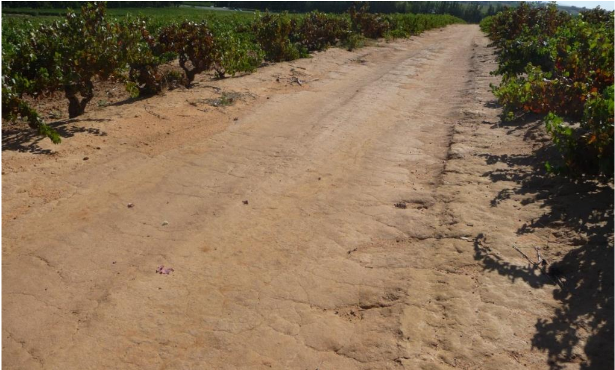
Figure 28 Loose soil flushed away by runoff from upper catchment, leaving a compact bare surface.
