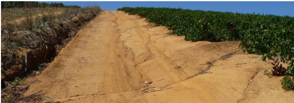
Figure 25 Road cambered concavely, inhibiting runoff from reaching the open ditch (right), instead causing erosion.
