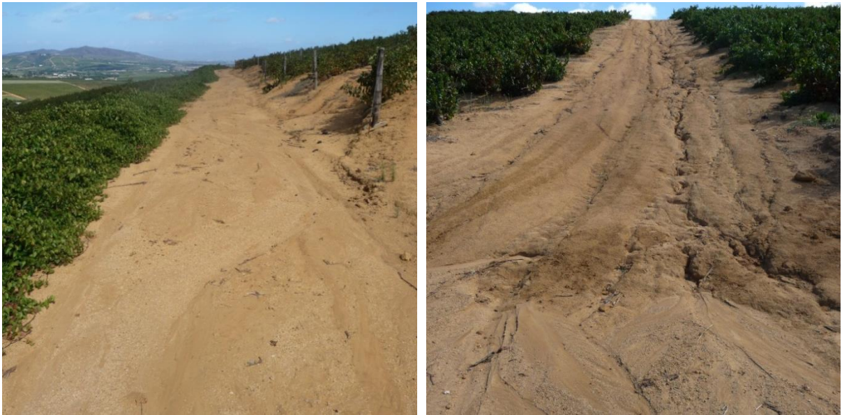
Figure 44 Left: Water safely transported on gently sloping ground towards the waterway. Right: Water which has escaped the earthen wall continues down a steep slope on the road between block 511 and 611.
