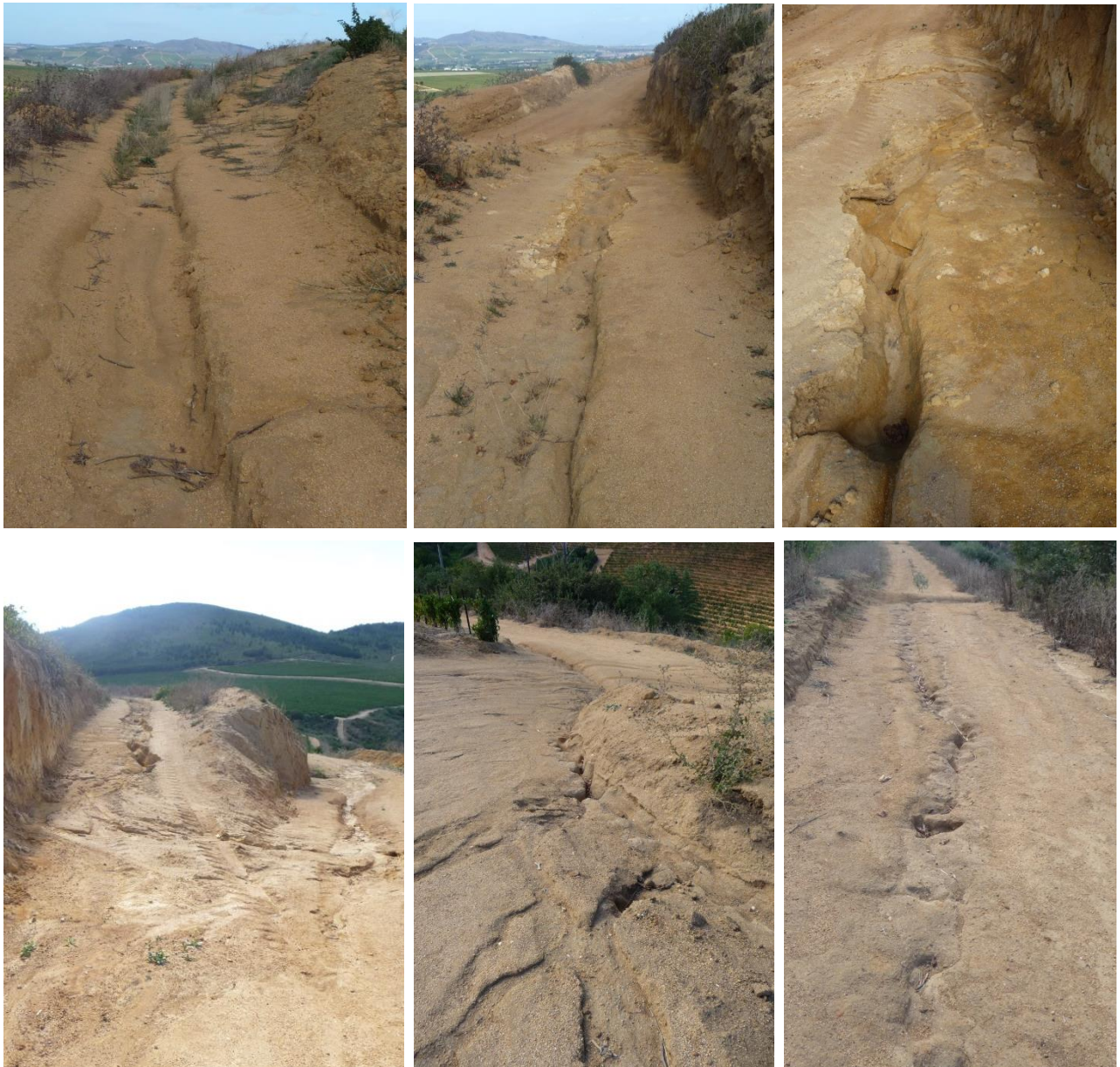
Figure 46 Runoff is initially transported safely in a man-made channel on a gentle slope (upper left). As the slope increase and additional runoff unite channel walls collapse (upper middle). The water is transported uncontrolled and takes a curve (upper right and lower left) continuing down the road (lower middle), eventually diverted into an area with natural vegetation (lower left).
