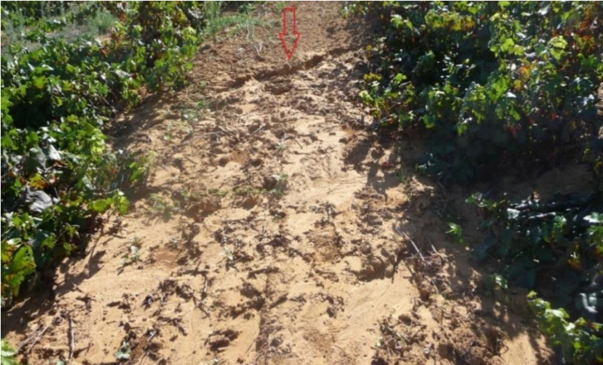
Figure 31 Signs of large water flow within vineyard block 308. Red arrow showing rill erosion.
