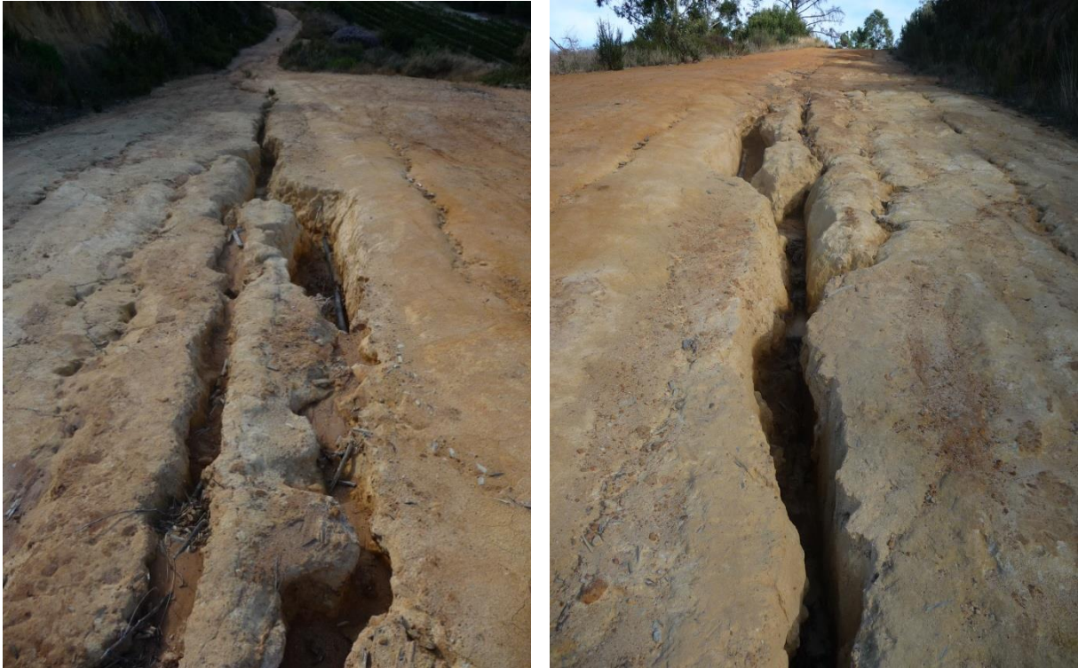
Figure 41 Left: Erosion seen from the top of the slope. Right: Erosion seen from the middle of the slope, looking upwards.
