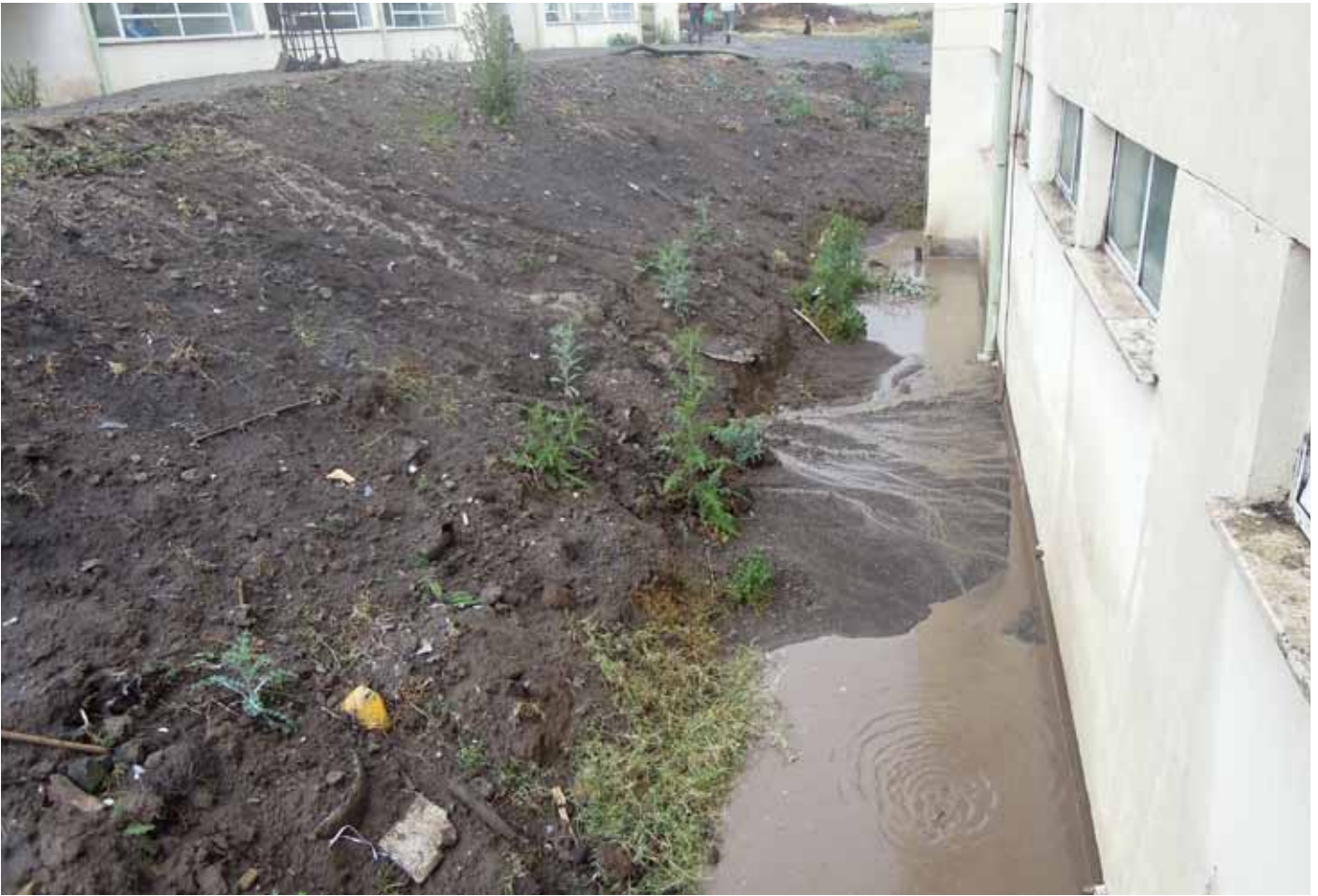
Soil and mud is moving down the hills and towards the buildings during rainfall.
