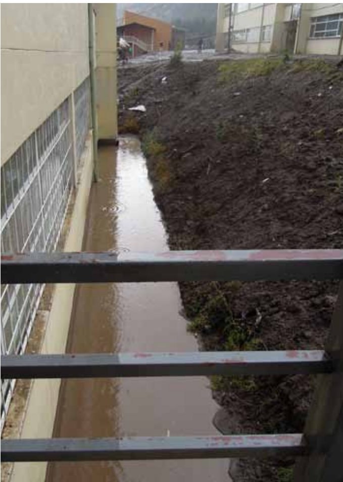
Water is accumulating too close to buildings during rainfall.
