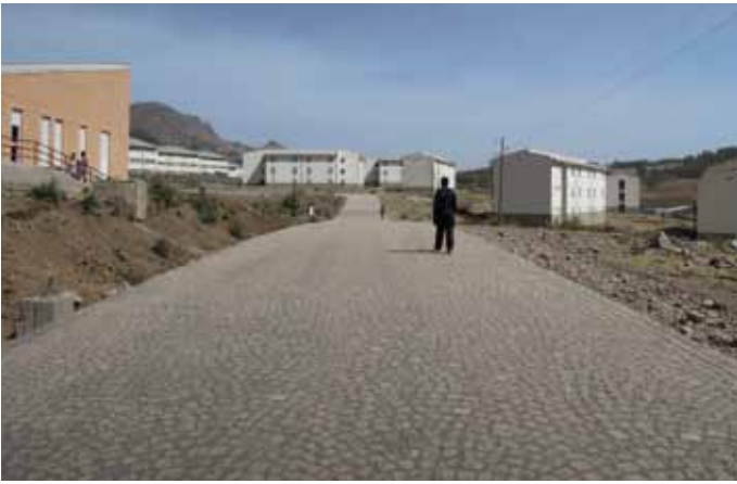
Cobble stones are the material that are planned to be used on all the roads within the site.
