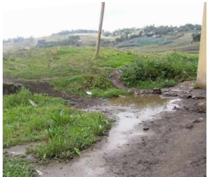
Grass, mud and water at bit too close to the buildings in the female residential area.
