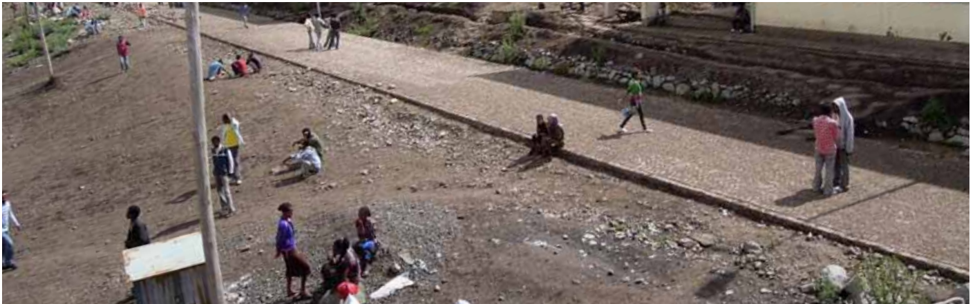
People are using stones and the edge of the newly constructed road to sit on.
