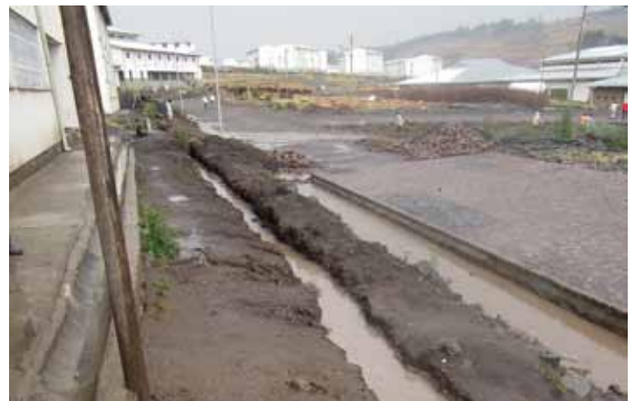
During rainy seasons large amounts of water are gathered in the unfinished and incomplete drainage system.
