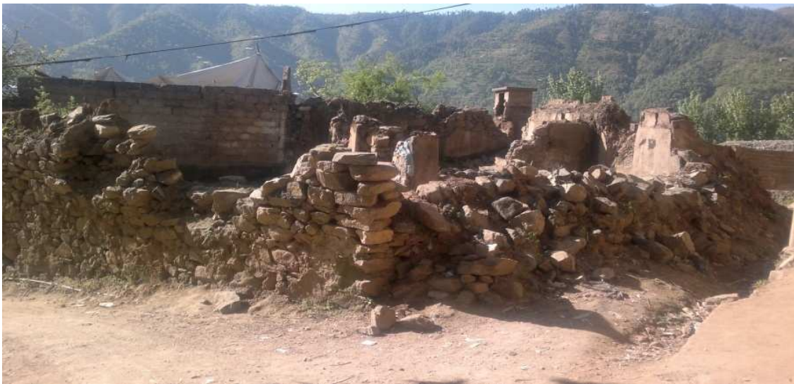
Fig 3 shows the house damaged in village A
