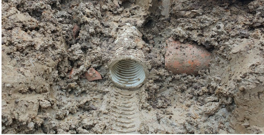
Figure 9. The picture shows how the new drainage pipe cuts through the old brick pipe in plot 7. Photo Linnea Berggren Sjögård
