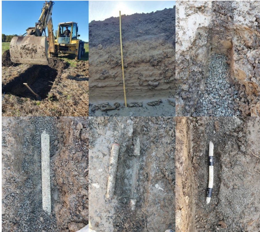
Figure 5. Pictures showing the excavation of the pipes in chronological order. Above left: excavation machine, mid above: soil profile, right above: the soil sample has been taken. Below left: exposed pipe, mid below: 40 cm of pipe cut off, right below: the joint pipe. Photo: Linnea Berggren Sjögård
