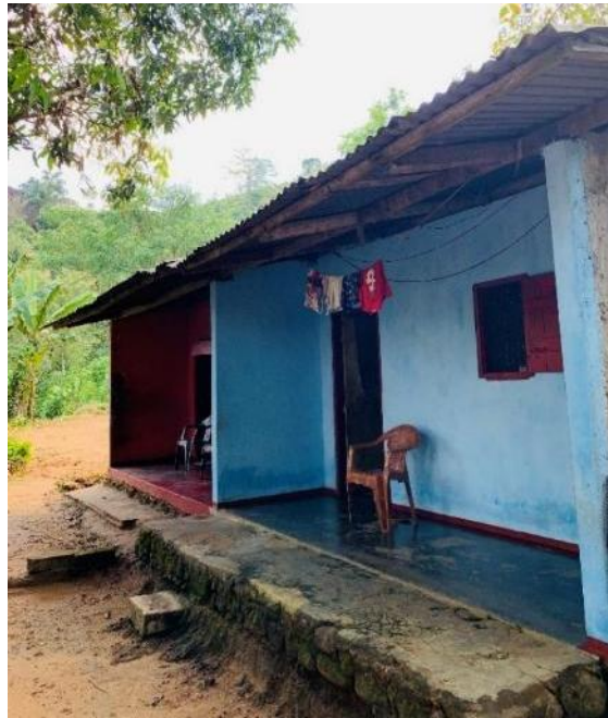
Figure 6 Exterior of a line room in a tea estate where workers live, featuring a small space, shared walls, and small windows, Thelbedda. 23/02/25, photograph by author
