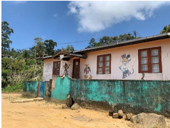
Figure 7 Exterior of an estate daycare center with aged walls and basic structure with fewer facilities, Haputale. 13/02/25. photograph by author
