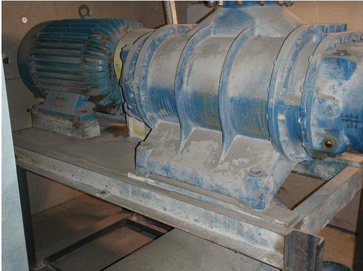
Figure 4.2-2 High pressure/volume blower installed inside a soundproof house. The blower was found in-house and was checked according to Cementa AB standards. Despite the fact that the blower is old vibrations in bearings were within an acceptable range. Normally when blowers are standing still for years in industrial environments damage occurs to the bearings (Larsson, 2008).
