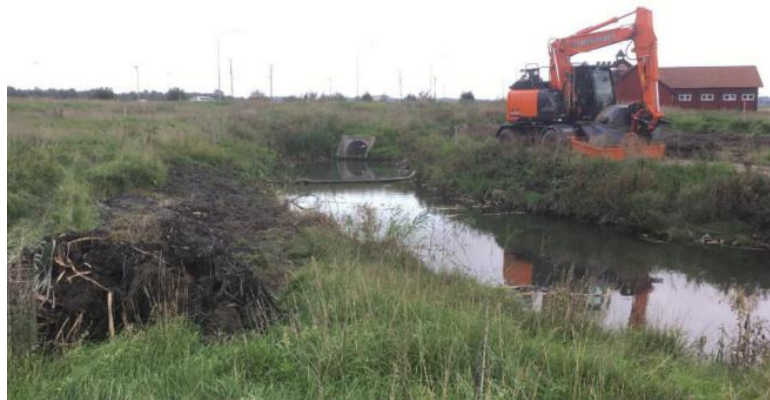
Figure 16. UW-Design allowing for Heavy Machine Access (photo: Jonas Andersson, WRS).
