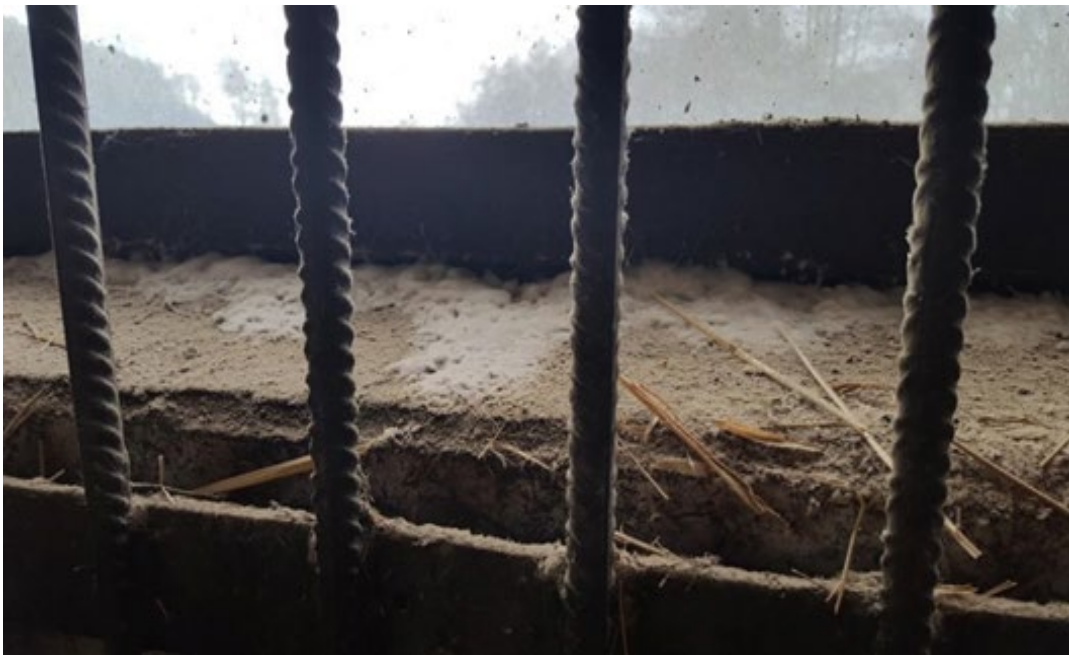
Figure 3. Mould on the windowsill close to where straw bales were kept. Photo: Jasmine Lindholm
