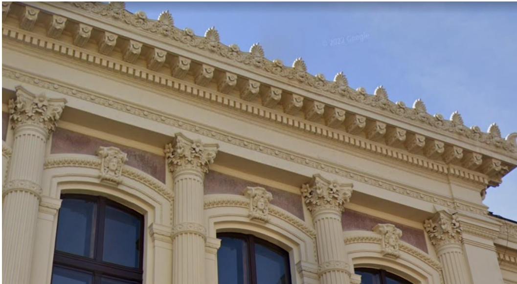
Figure 20. Face of a building along Östergatan, Malmö. This building is one of the most lavishly decorated building covered with organic forms found in different parts of the façade such as the Corinthian capital, human-relief keystone, and entablature. Organic forms such as these were not traced.
