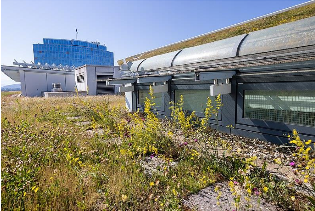
Figure 6. Green roof at WIPO headquarters in Geneva, Switzerland (Emmanuel Berrod 2021) (CC BY-NC-ND 2.0)
