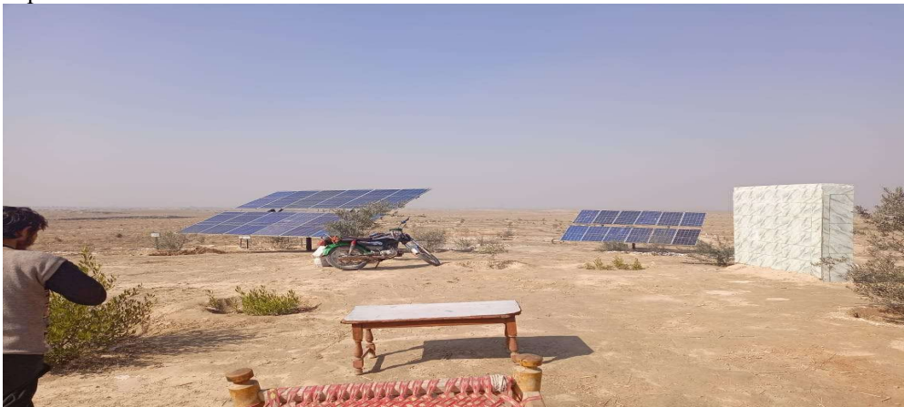
Figure 10: Usage of solar panels for tube wells at the plantation site
