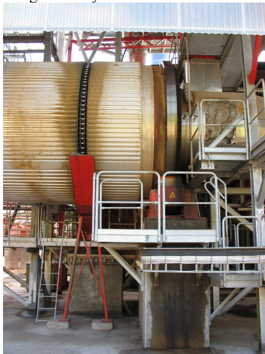
Figure 3.9. The inflow section of a rotating drying drum in a briquette- and pellet facility (Photo Johan Karlhager)
