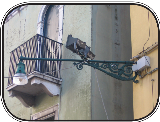
The existing wall brackets need to be shielded off to prevent light pollution and disturbance.
