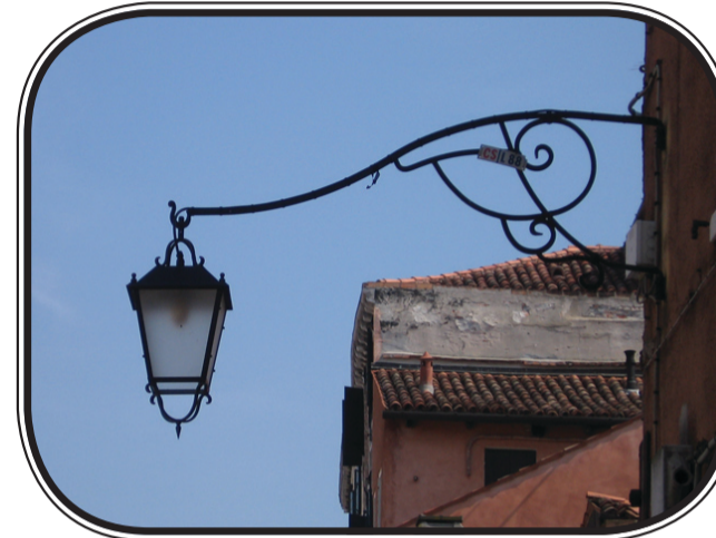
This type of luminary used to be connected with hooks.
