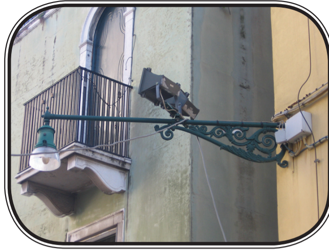
The most commonly used wall brackets in Venice, here with floodlights placed on the bracket.
