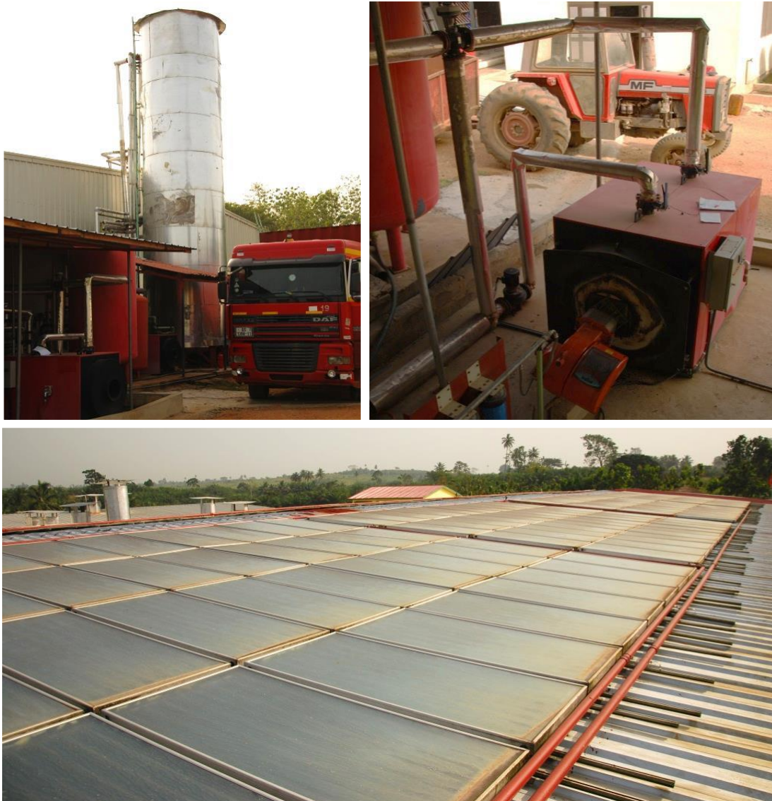
Figure 4.5: Heat storage tank, kerosene boiler and solar panels
