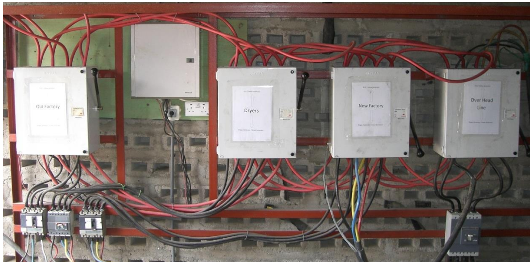
Figure 4.3: Electrical main loads. From left: Old factory, Dryers, New factory, Overhead line
