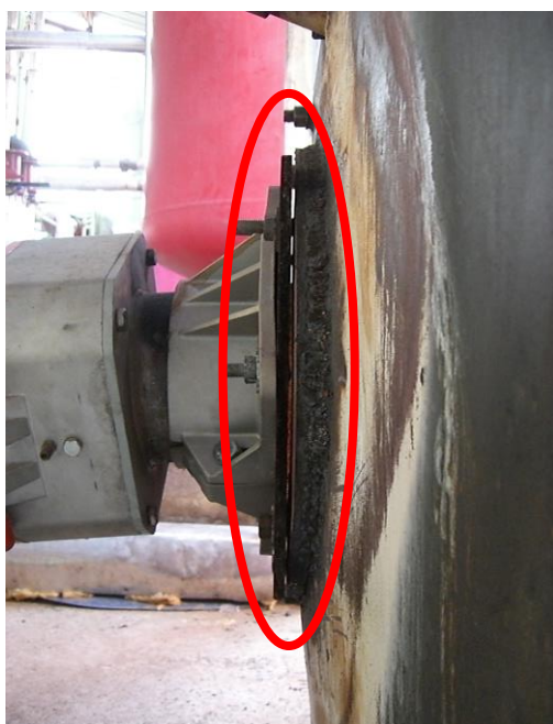
Figure 8.3: Leaky burner intake of kerosene boiler
