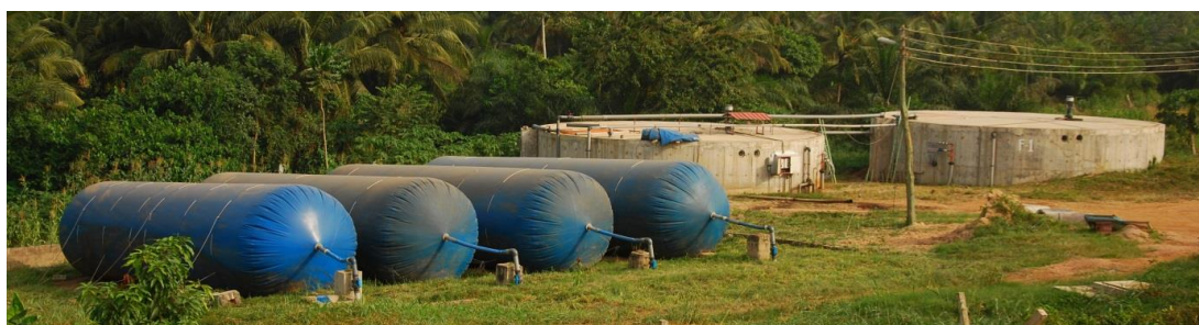
Figure 4.6: Fermenters and gas storage balloons of the biogas plant
