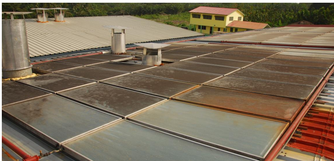
Figure 8.7: Dirty solar panels around the chimneys of the dryers on the east side of the roof
