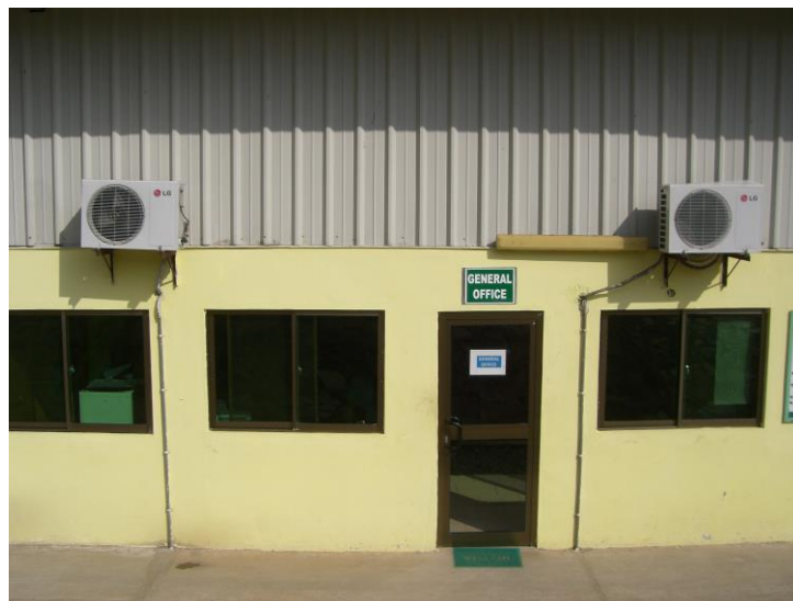
Figure 8.2: Placement of condensers for general office's cooling machines
