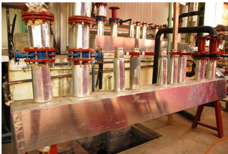
Figure 8.8: Two new connection boards for the heat system, with return (atop) and supply
