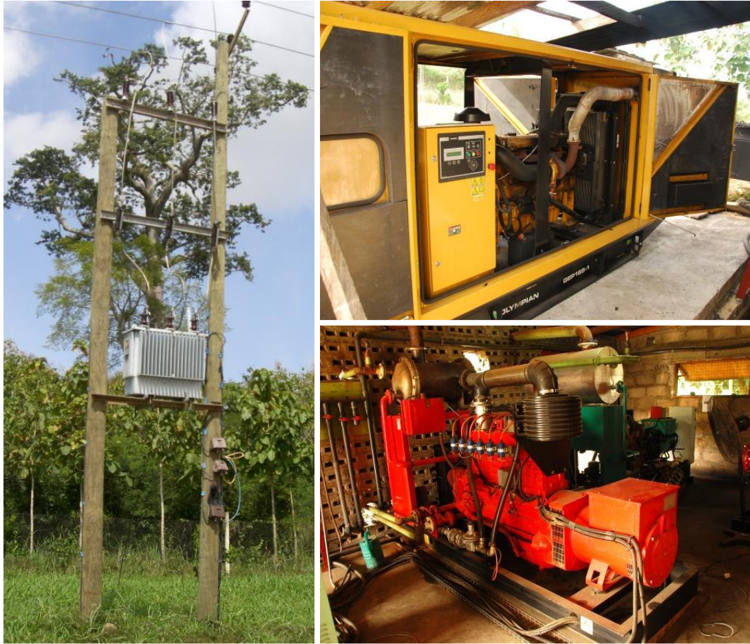
Figure 4.2: Transformer, diesel generator (yellow) and biogas CHP (red)
